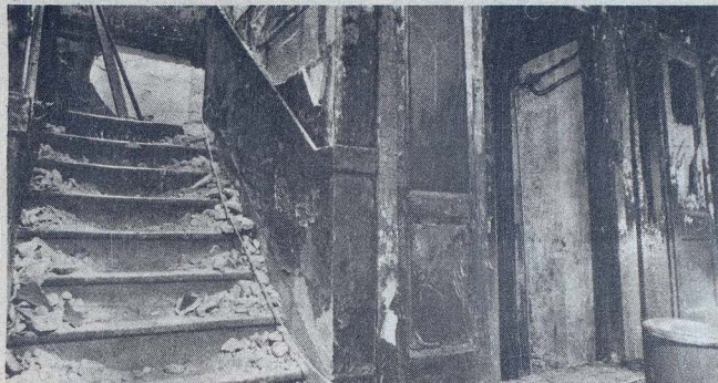
BADLY BURNT BASEMENT -Charred doorways and blistered walls provide evidence of the fire that put the heat on the bottom floor of the Traveler's Hotel. The upper stories received only smoke damage.
