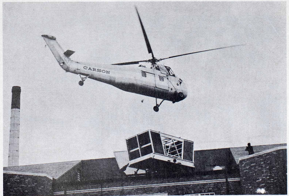
Operation air lift air conditioning took place on the NMSC campus this spring as a part of the complete air conditioning of the Student Union, Violette Hall, Baldwin Hall, Science Hall, Pickler Memorial Library. Carson Helicopter Service, Inc. of the state of Pennsylvania is pictured lifting a 5,200 lb. cooling tower into place on the roof of Violette Hall. The helicopter lifted numerous air handling units and auxiliary parts for the building tie-in system, which is nearing completion.
