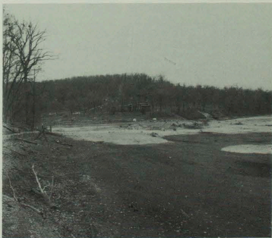
These pictures were taken in 1961 while the leak in the lake's dam was being repaired. The lake was drained to allow bulldozers onto the dry bottom to do the necessary dirt work. The empty lake exposed many tree stumps and gave members the chance to remove debris that could interfere with successful fishing.
