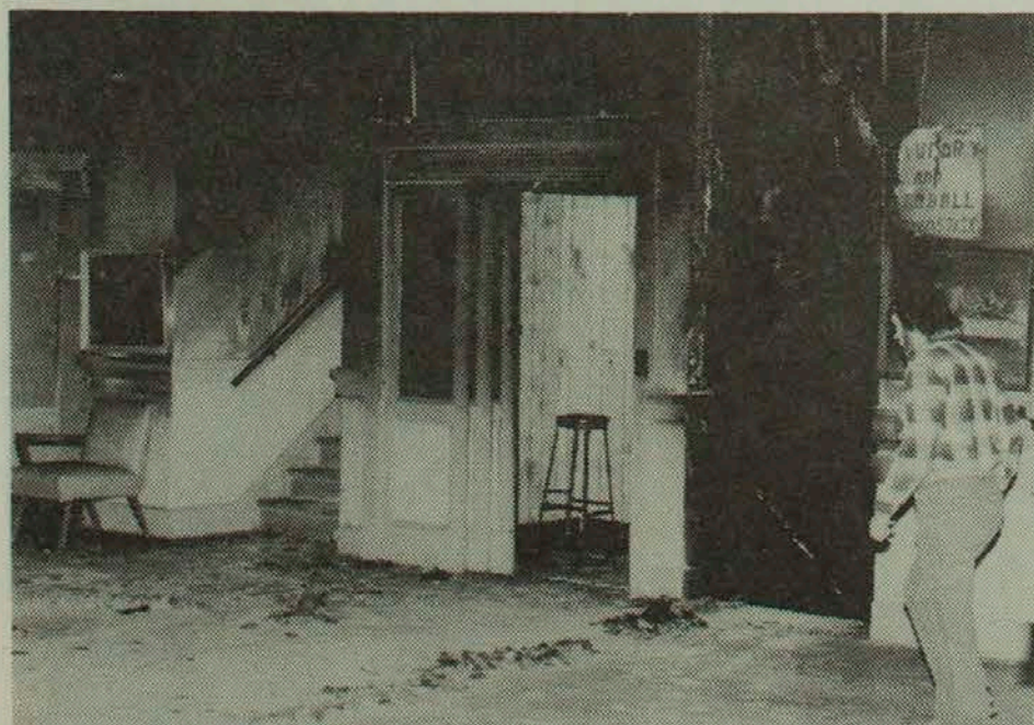
The first floor of the hotel suffered severe smoke damage in a fire in 1981.
