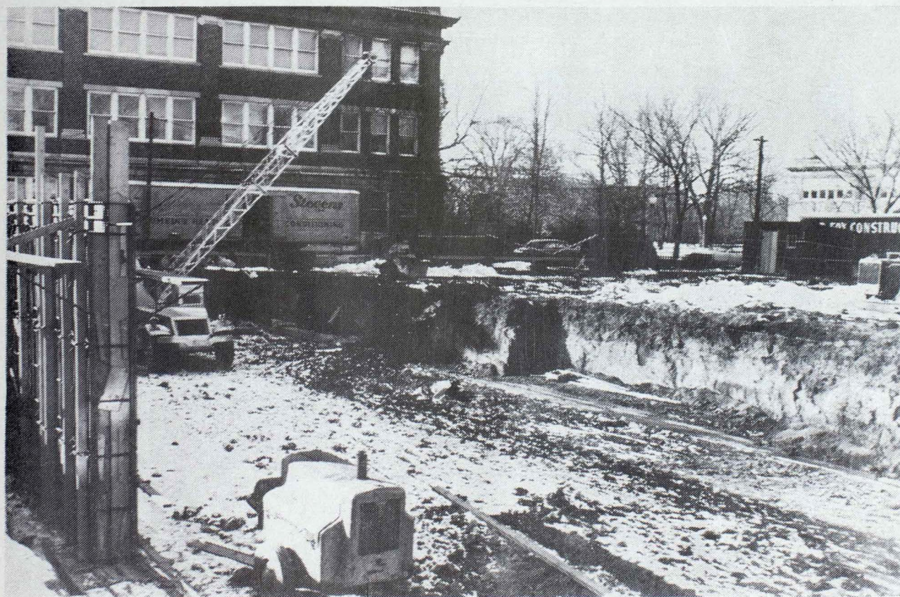
Excavation for Brewer Hall, Men's Dormitory Being Constructed Adjacent to Nason Hall
